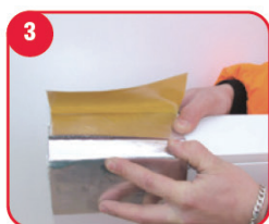
3 Wrap around service to a tight fit
